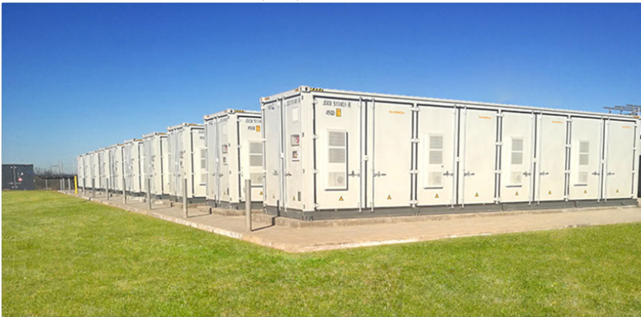
Figure 1- Battery on Slab
