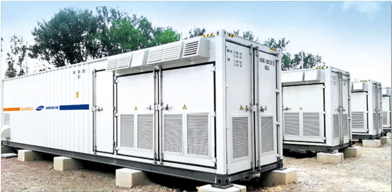
Figure 2- Battery on Pier
