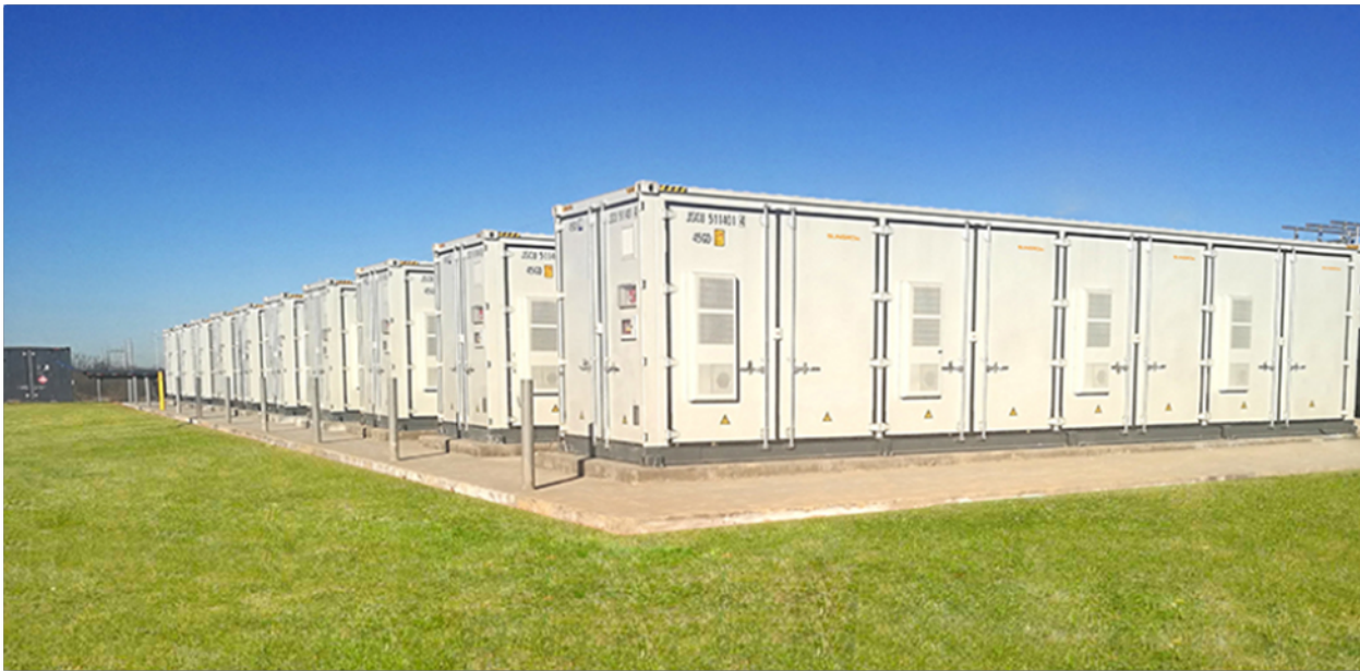
Figure 1- Battery on Slab
