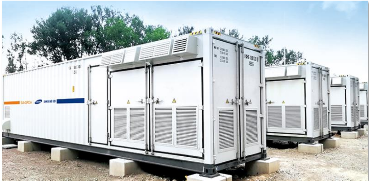
Figure 2- Battery on Pier
