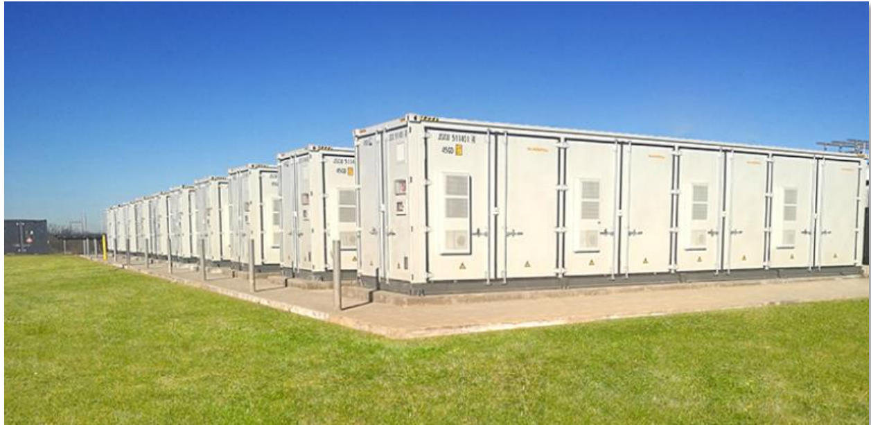
Figure 1- Battery on Slab
