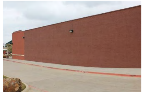
Figure 7-4 Blank Wall- Prohibited
