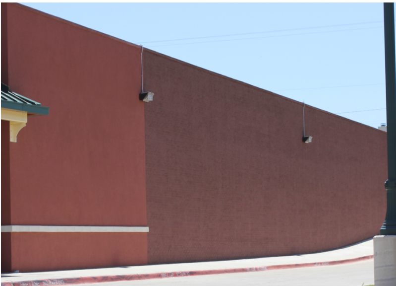
Figure 6. Not permitted: No articulation along the façade
