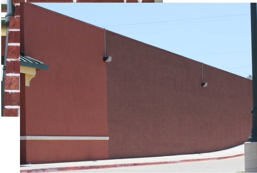
Figure 4. Not permitted: No articulation along the façade
