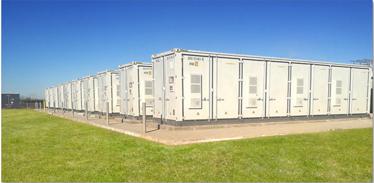
Figure 1- Battery on Slab
