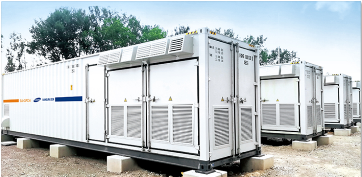
Figure 2- Battery on Pier
