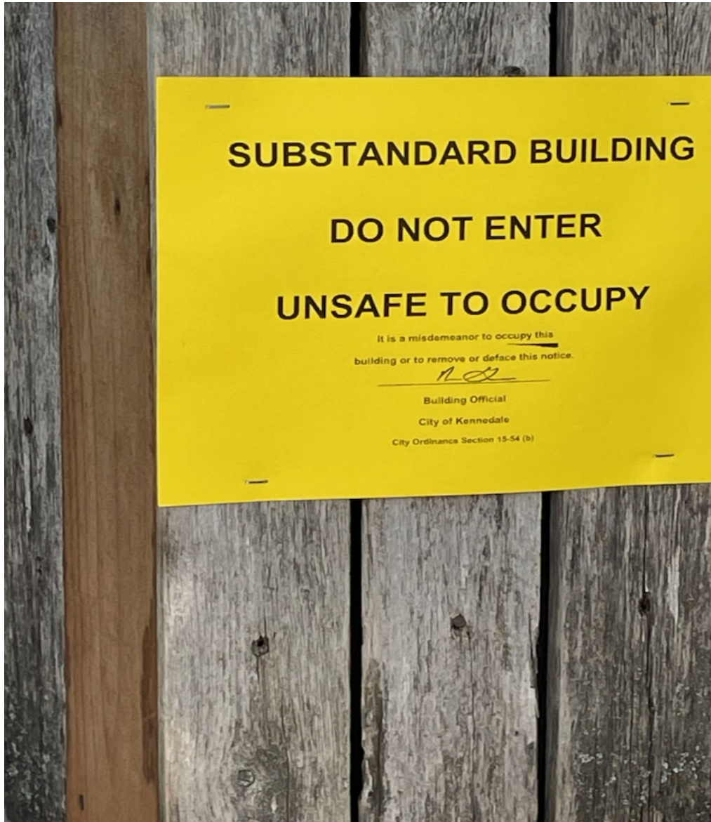
Notice Posted- Fence in Front of Property
