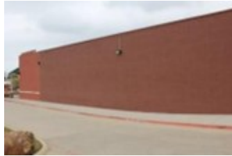
Figure 7-5 Blank Wall - Prohibited
