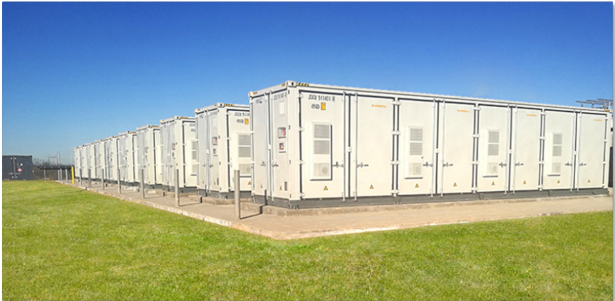
Figure 1- Battery on Slab
