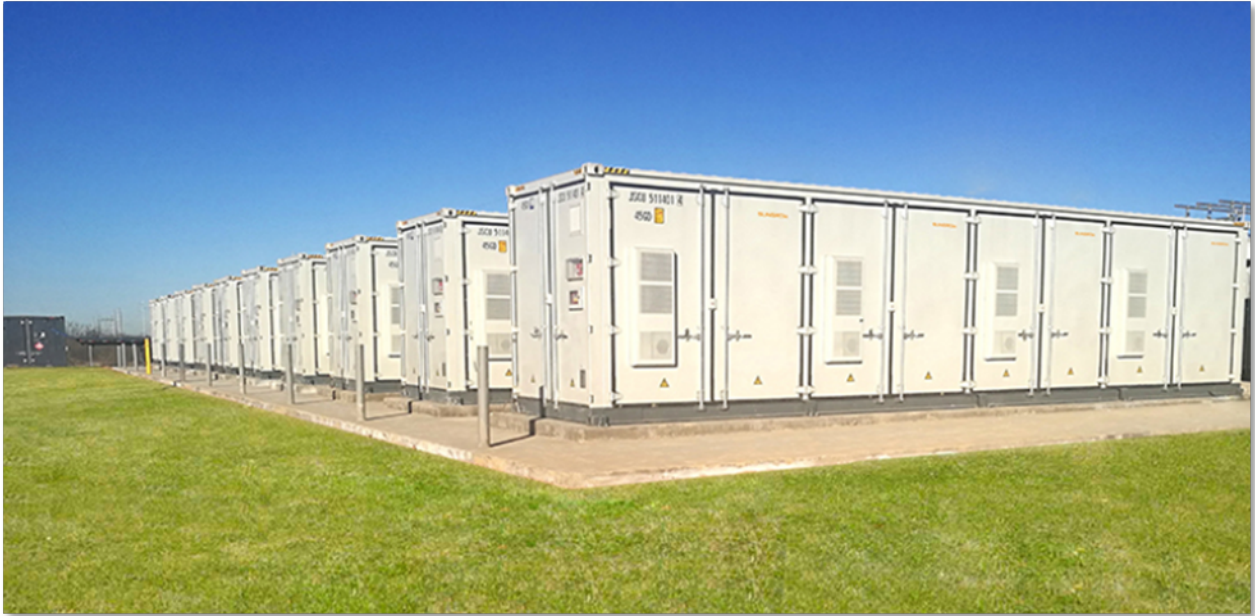
Figure 1- Battery on Slab
