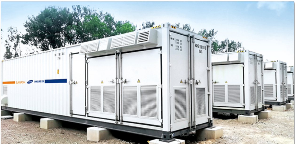
Figure 2- Battery on Pier
